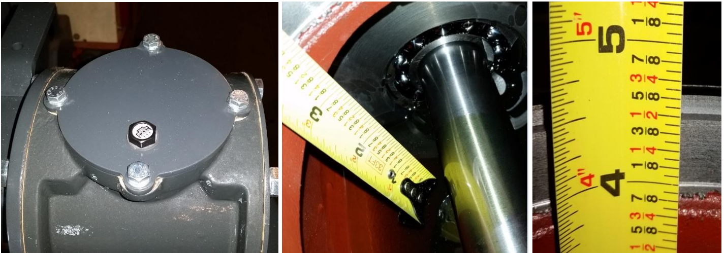
Figure 12 - oil level is 4-5/8" down from the top of the gear box
